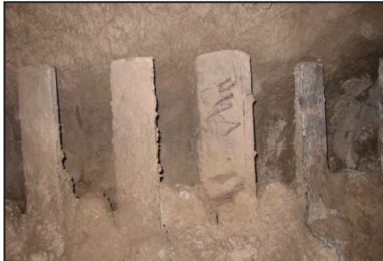
Condition of the pug mill blades in service
